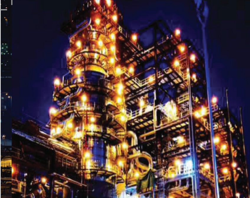
AGIP Kashagan Refinery Project, Atyrau, Kazakhstan
